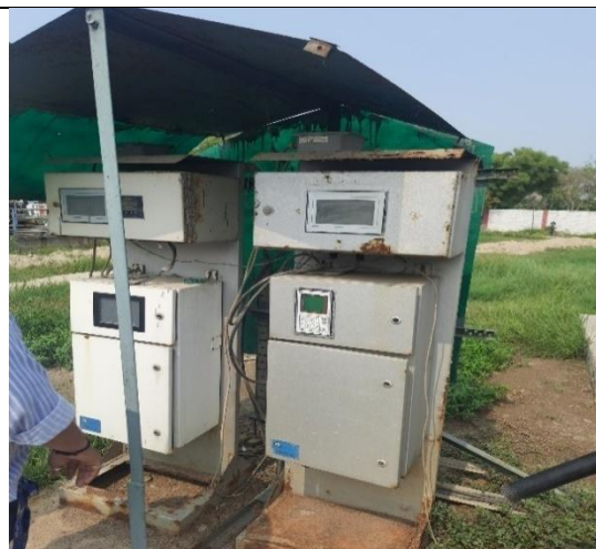
OCEMS installed at CETP Inlet (Defunct)
