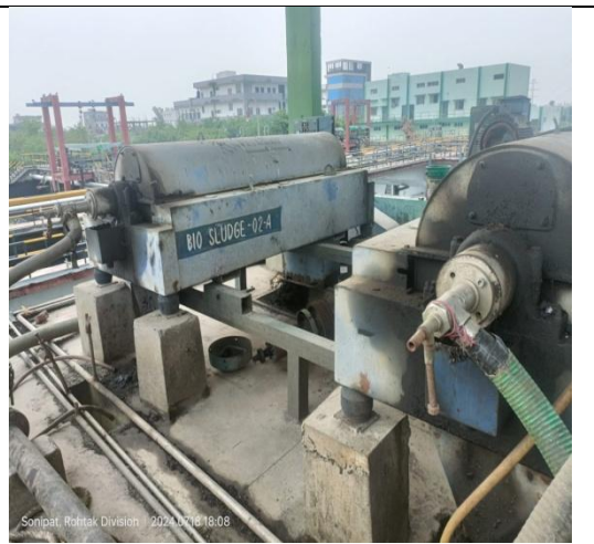
Sludge dewatering unit
