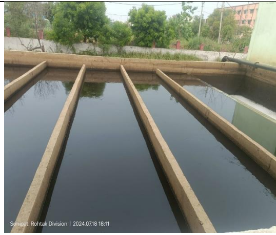
Chlorine Contact Tank
