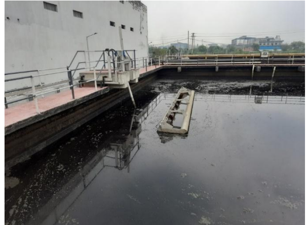
Decantation in SBR Tank
