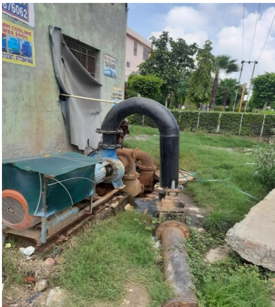
Intermediate storm water pumping station at Phase-I
