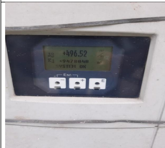
Flow meter installed at CETP Outlet
