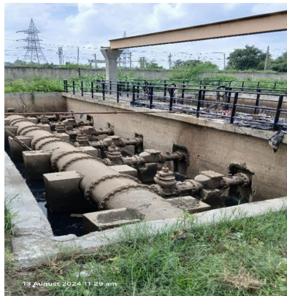
Main storm water pumping station at Phase-III
